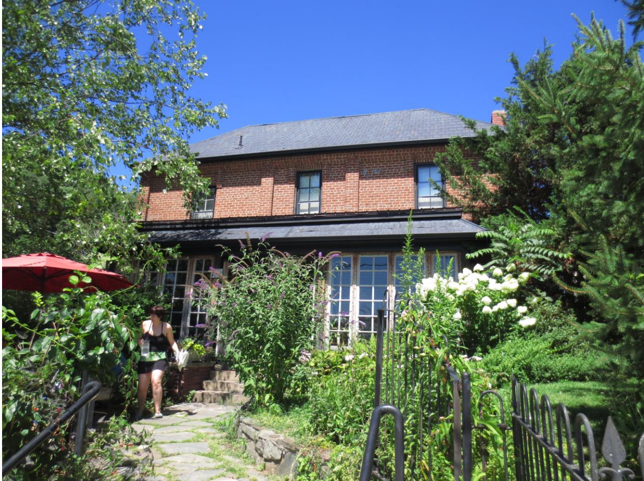
The Watauga County Jail features important masonry details on its primary elevation. Patching of second-floor masonry using Portland cement and other materials mars the historic appearance of the masonry and poses a risk to its stability. Photo courtesy of Eric Plaag, 2015.
