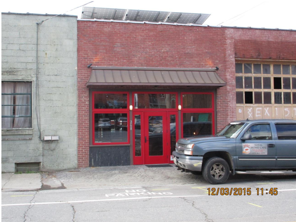
The solar array on the rooftop of this Howard Street property was installed too close to the front of the building, so that it is easily visible from the street level in front of the primary elevation. Such additions should be positioned toward the tertiary elevation to avoid degradation of the historic character of the District. Photo by Carson Hamilton, 2015.
