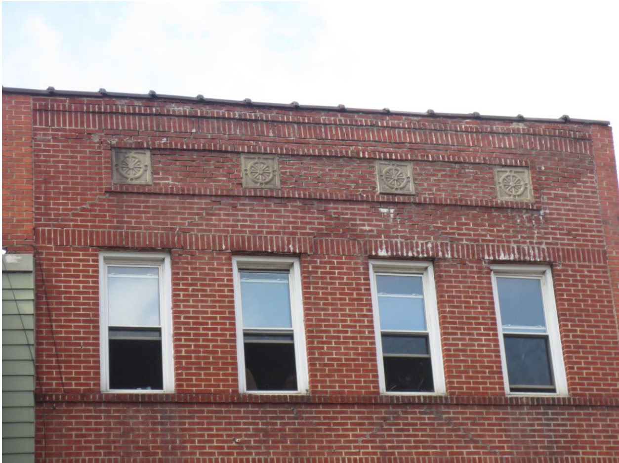
This West King Street property has suffered from poor attempts at re-pointing the masonry between the roofline and upper story windows. Photo courtesy of Eric Plaag, 2013.
