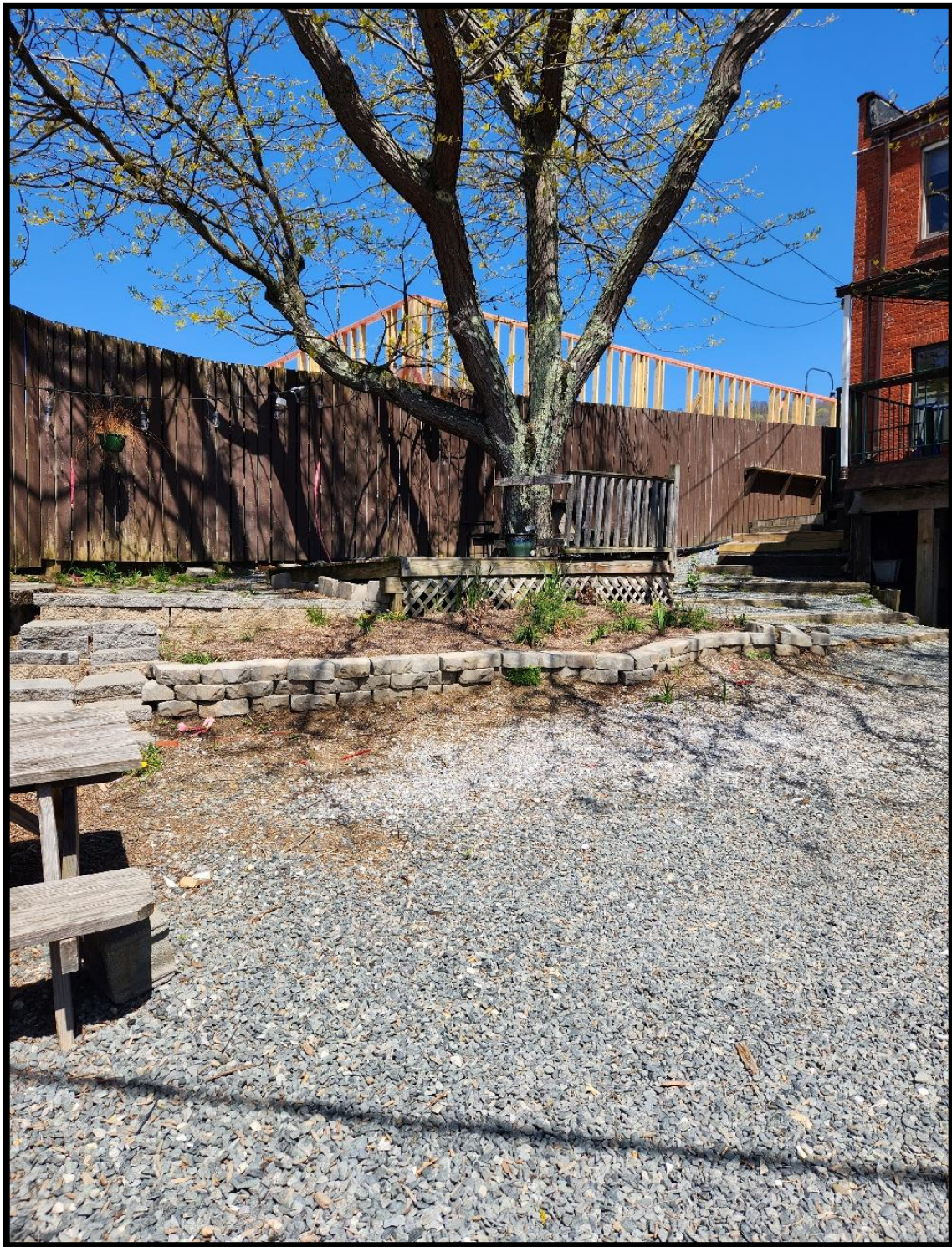
Figure 3: SEBB Eroding retaining wall #1 – April 18, 2023
