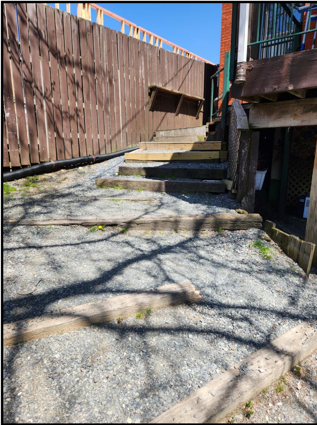
Figure 5: SEBB Deteriorating steps to existing deck – April 18, 2023.
