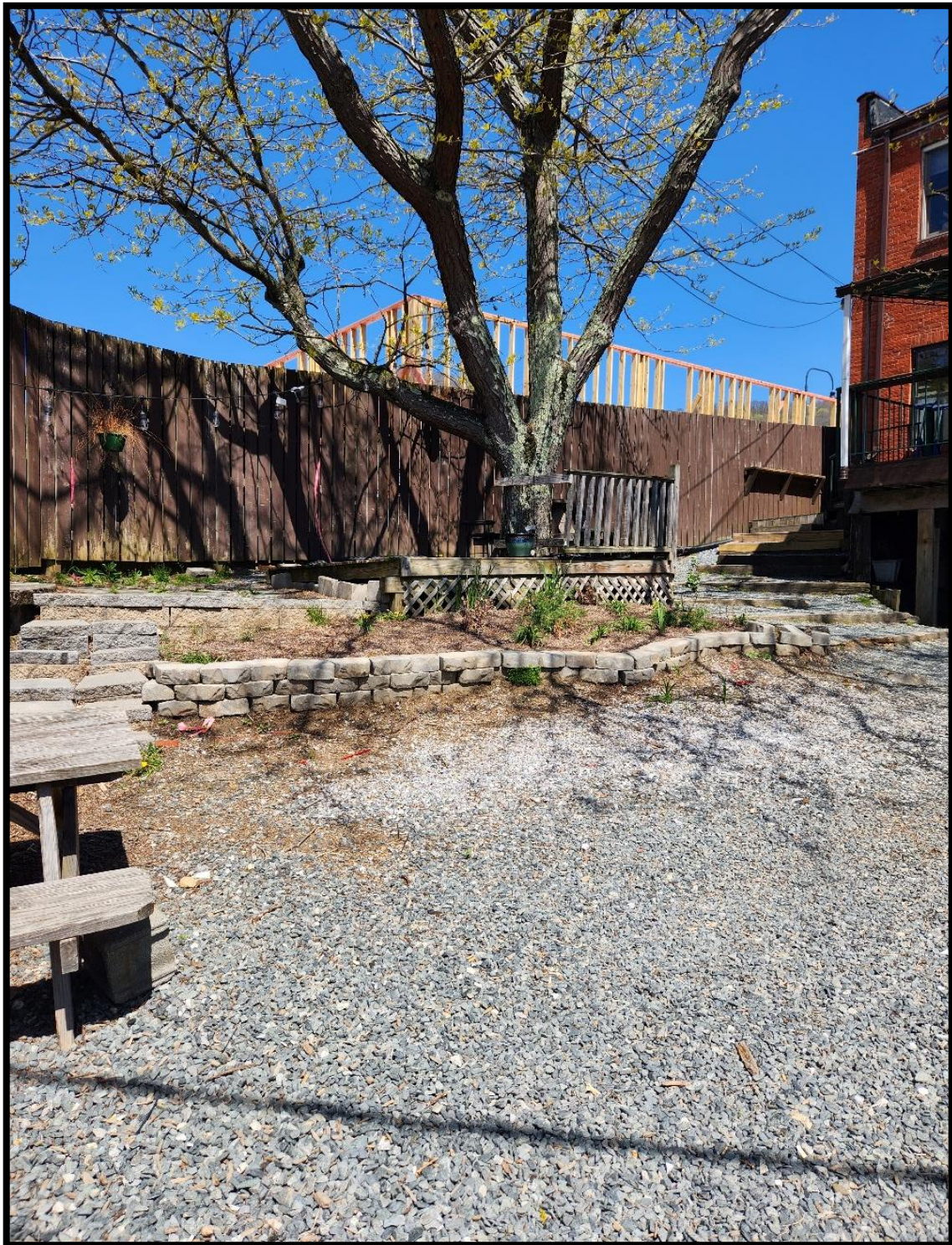
Figure 3: SEBB Eroding retaining wall #1 – April 18, 2023
