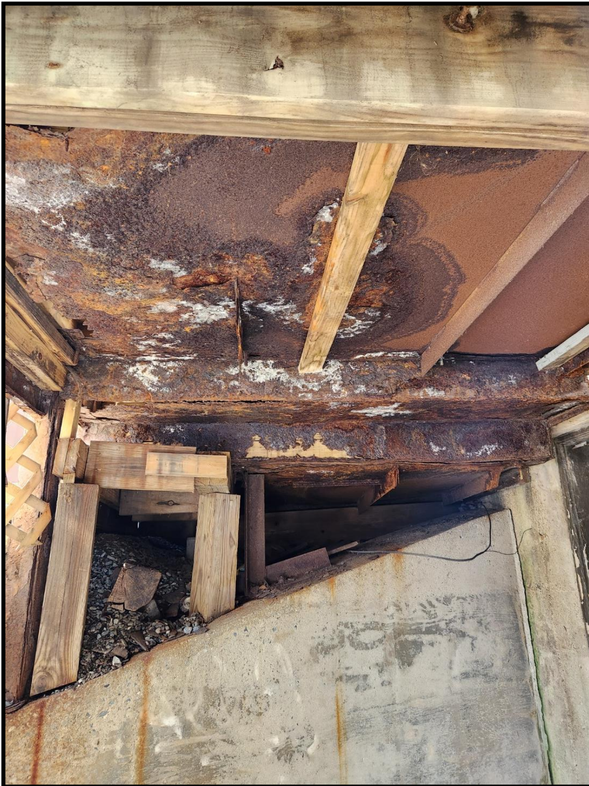
Figure 7: SEBB Underside of existing deck with extensive rusting and disintegration – April 22, 2023
