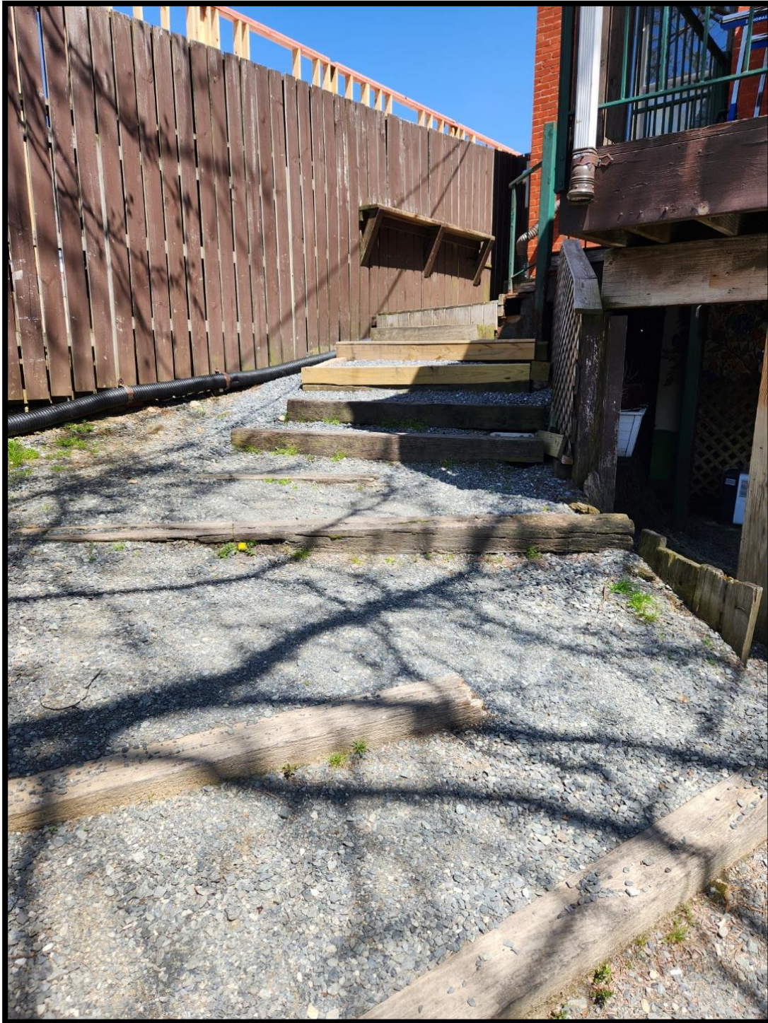
Figure 5: SEBB Deteriorating steps to existing deck – April 18, 2023.
