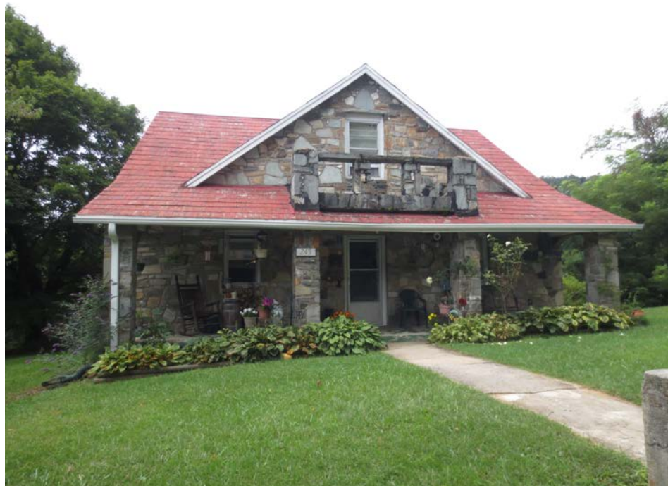
The use of tar as a flashing material, as seen around the second story porch of this historic and otherwise very attractive Boone residence, can damage original masonry and is unsightly. Photo courtesy of Eric Plaag, 2013.
