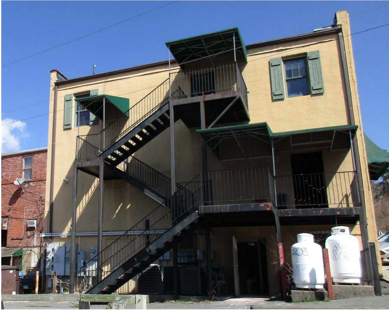
Updated fire escapes, like this one on a King Street building, should be located on a tertiary elevation not visible from streets adjacent to the primary and secondary elevations. Photo by Eric Plaa, 2016.
