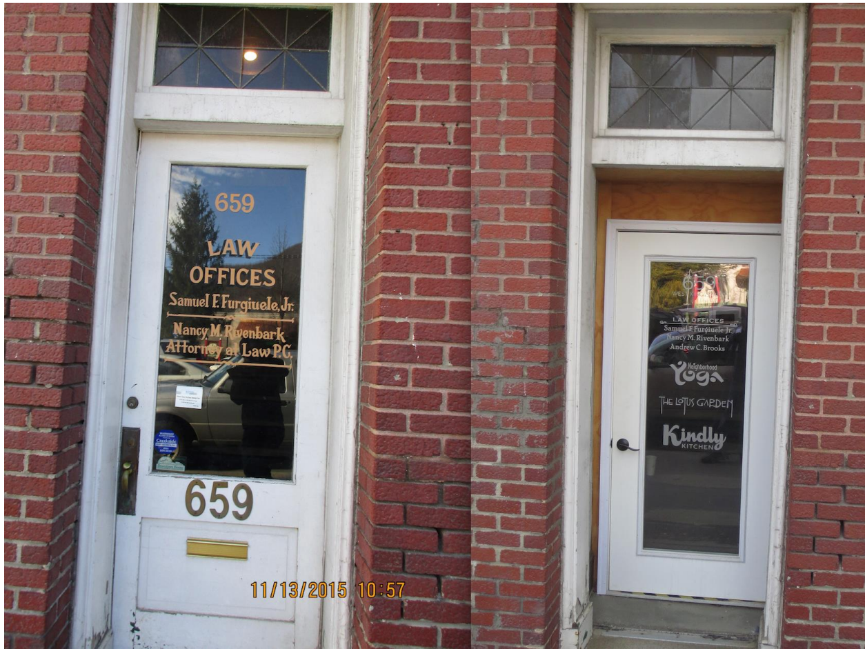
Original door configurations, like the one seen at left in November 2015, should never be abandoned for modern, historically inappropriate treatments like the one seen in the same doorway at right in January 2019. Images by Paul Fuller (left) and Eric Plaag.
